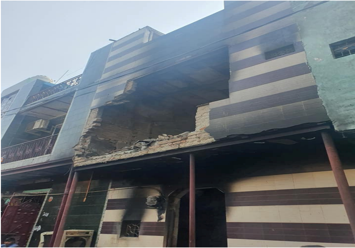
A damaged house in the riot affected area (Photo taken by the chairman of the fact-finding committee)
